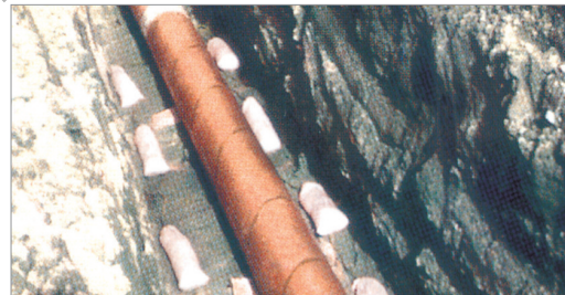
지하배관용 매설 MAGANODE MAGANODE Installed for Underground Pipeline
