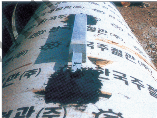
배관에 설치된 ZANODE / ZANODE Installed on Pipe
