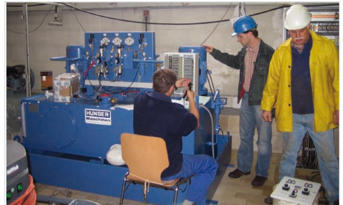
Installation of cylinders, hydraulic power unit and execution of the piping at the hydro electric power station Wallstadt, Germany
